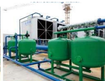
Chemical plant side water filtration
