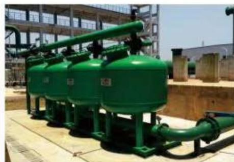
Coating factory side water filtration
