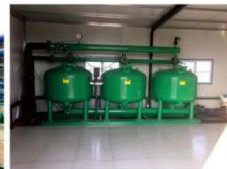
Filtration system for irrigation
